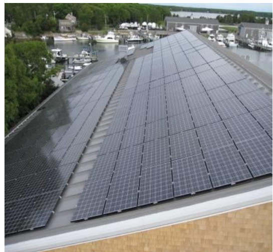
Roof Top Solar
