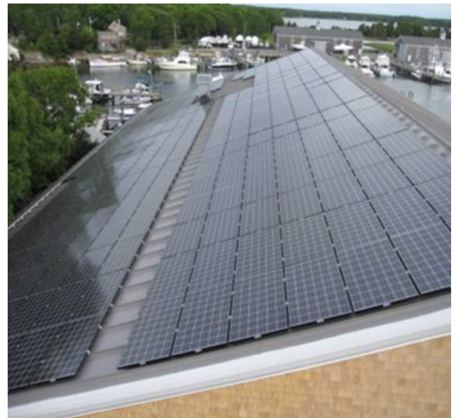
Image 33: Roof Top Solar
