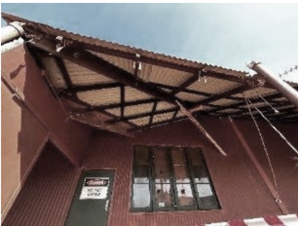
Figure 73: Damaged verandah canopy timbers
