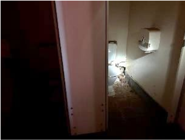
Figure 86: Damaged wall in toilets
