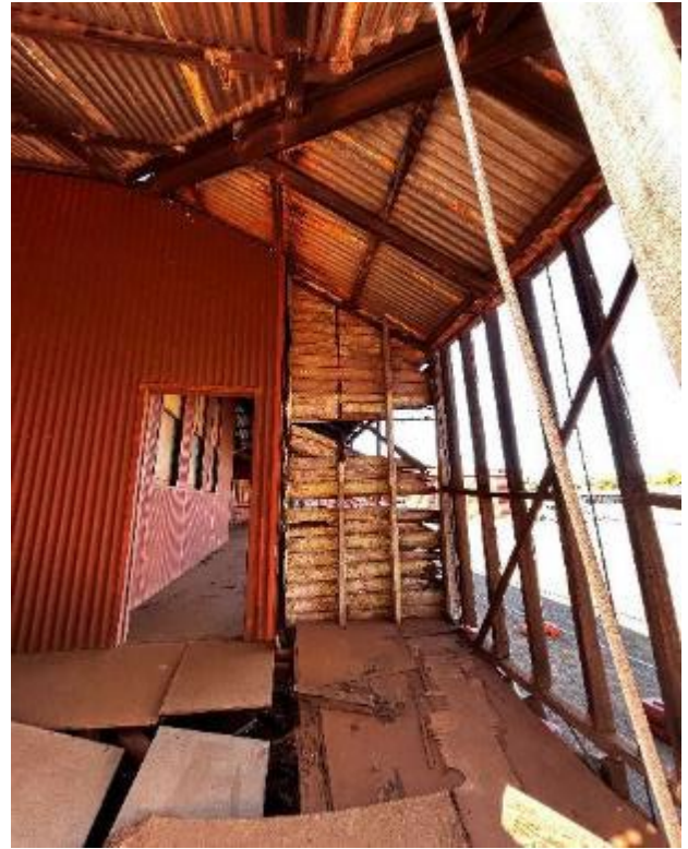
Figure 69: Collapsed verandah and loss of cladding materials
