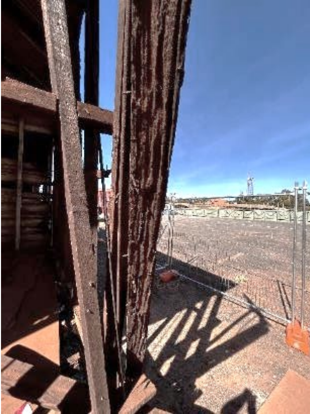
Figure 82: Termite damaged verandah timbers
