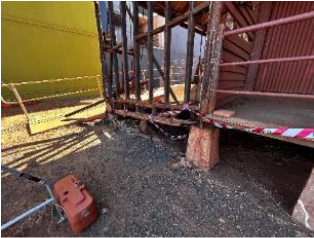
Figure 67: Collapsed northern verandah
