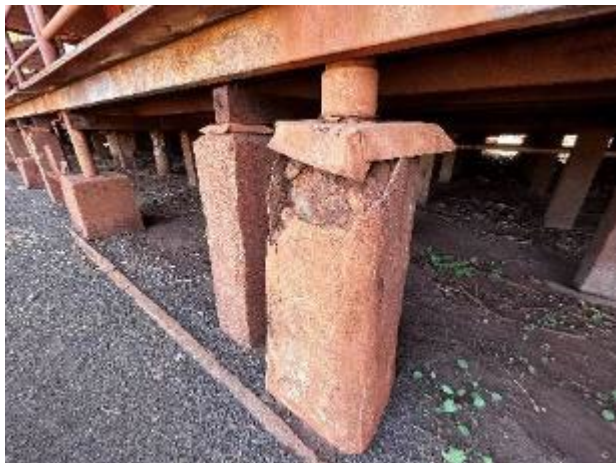
Figure 66: Typical concrete damage to stumps
