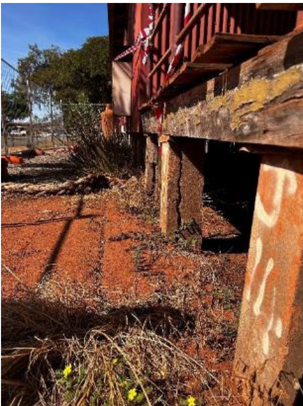
Figure 78: Damaged stumps and verandah facing plate
