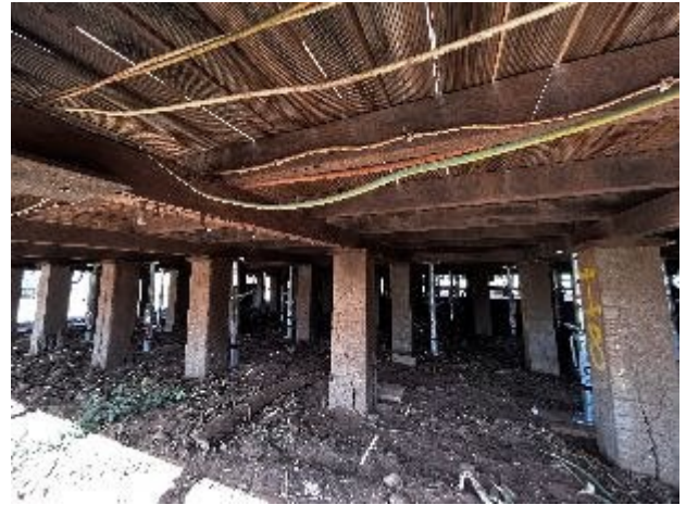
Figure 74: Unsafe wiring under the building
