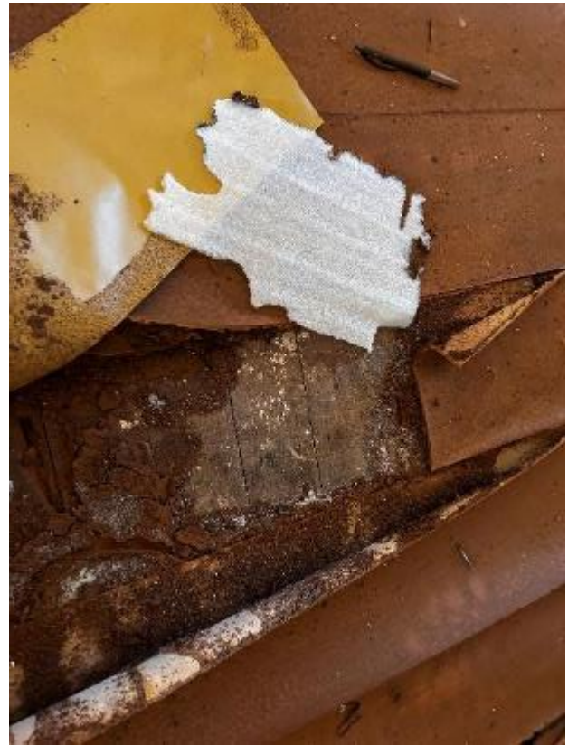
Figure 89: Damaged timber floor in Main Hall 2
