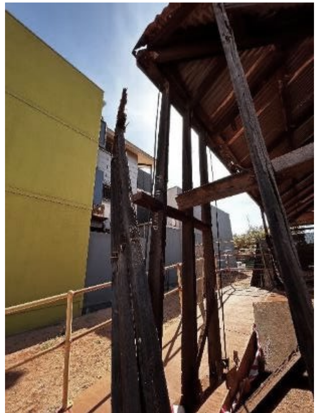
Figure 70: Damaged verandah timbers
