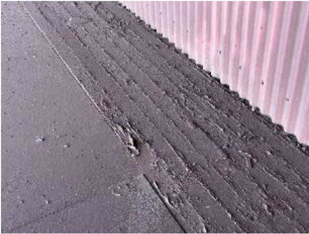
Figure 71: Deteriorating verandah timbers
