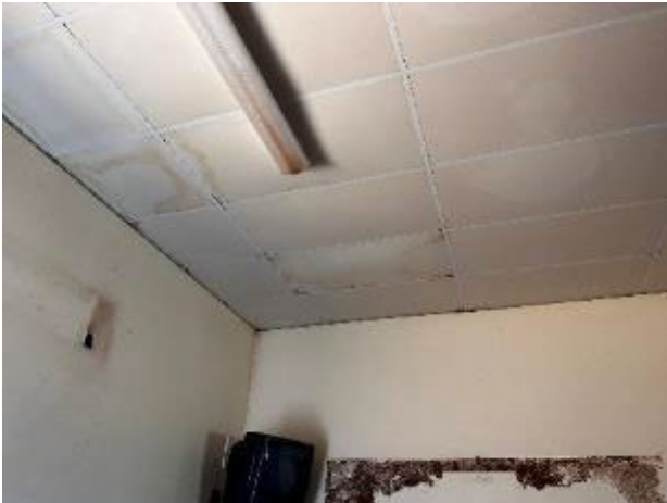
Figure 91: Damaged suspended ceiling in Main Hall 2
