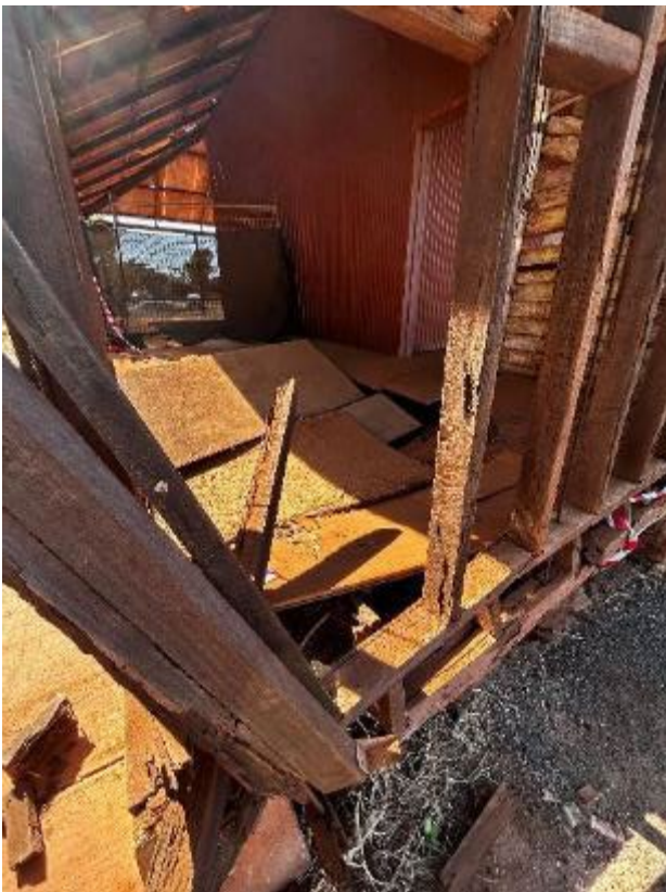
Figure 68: Collapsed northern verandah
