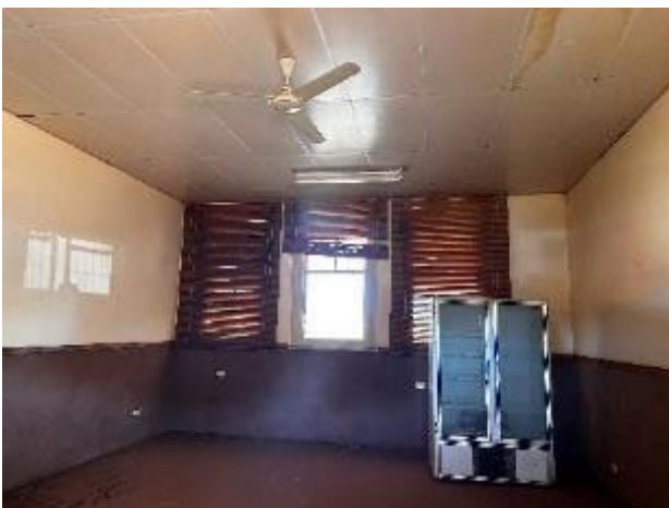
Figure 88: Damaged ceiling in Main Hall 2
