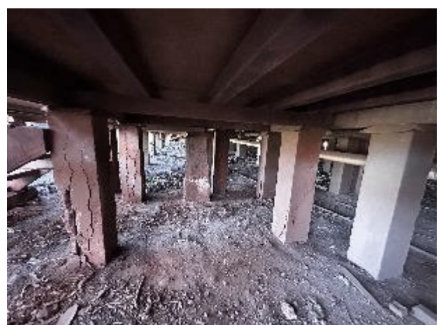
Figure 76: Damaged and replaced concrete stumps
