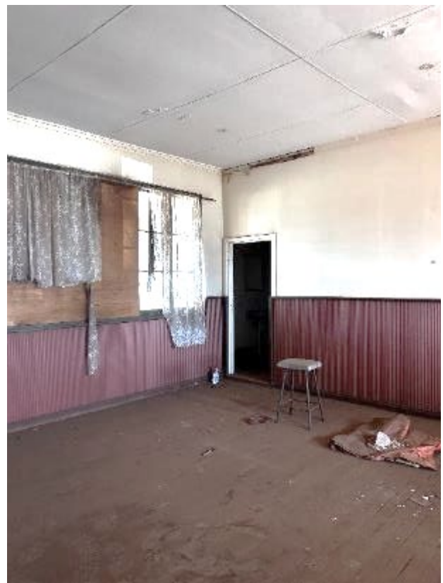
Figure 85: Boarded up window and damaged ceiling
