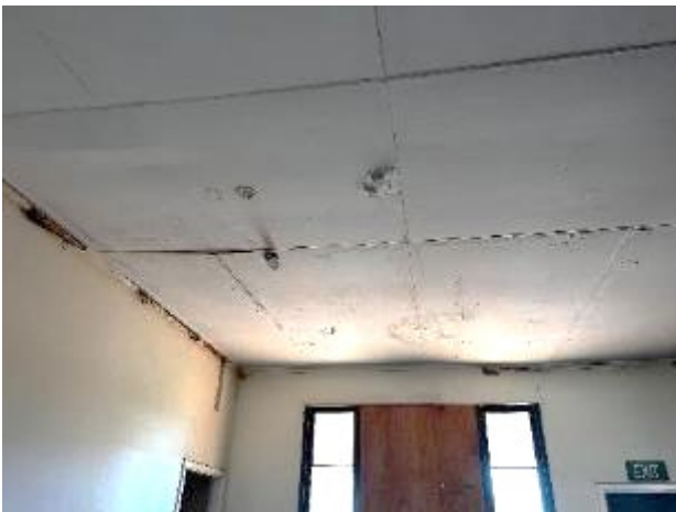
Figure 87: Damaged ceiling in Main Hall 1
