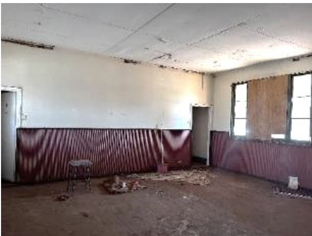
Figure 83: Damaged ceiling in Main Hall 1
