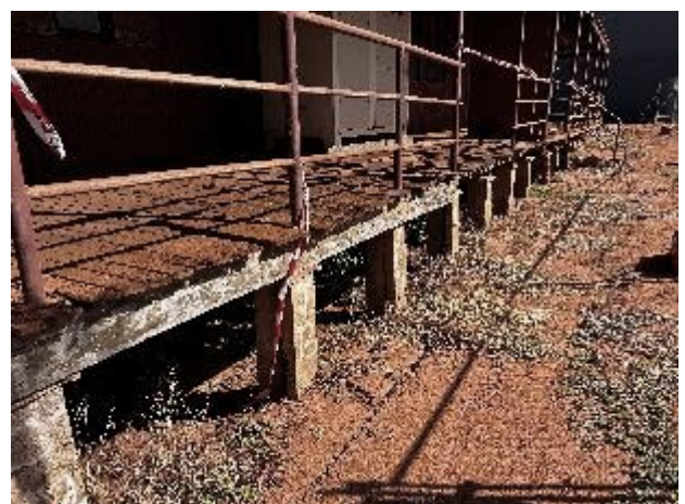
Figure 75: Verandah in poor condition
