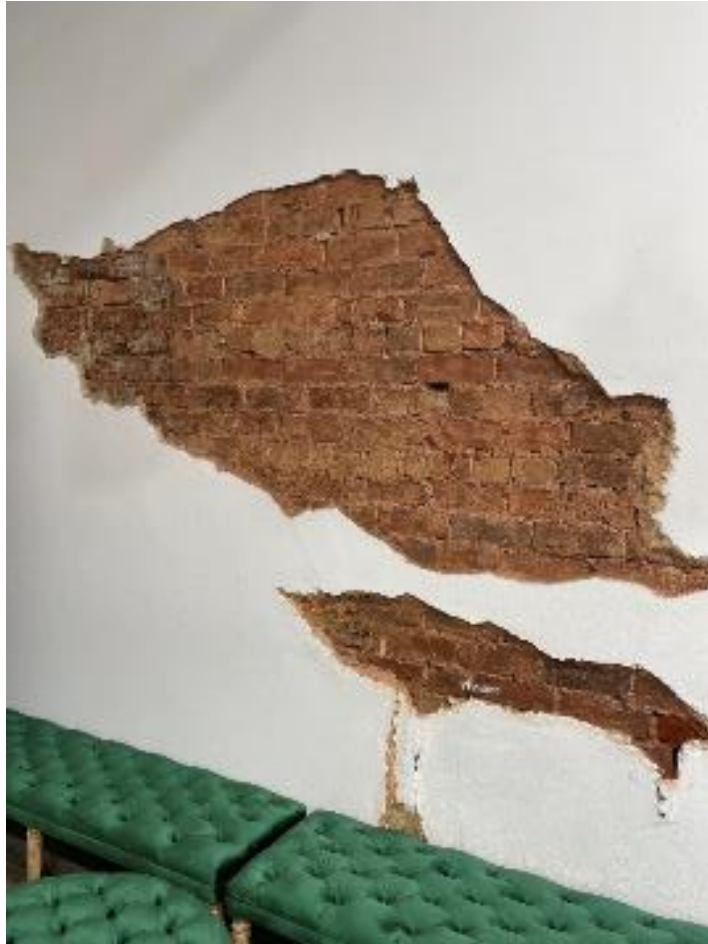
Figure 83. Detail view of No. 290 Damaged section of plaster render. It is unclear if this relates to historic rising damp or localised impact damage.
