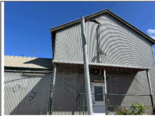
Figure 32. Though reflective of the era it was constructed, the building complements the industrial form of the site.
