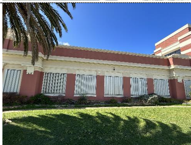
Figure 12. Providing a counterbalance to the dominant factory frontage, the single storey office building has a horizontal emphasis with a symmetrical presentation. The central entrance section is flanked by recessed wings which present with a rhythm of fenestration.
