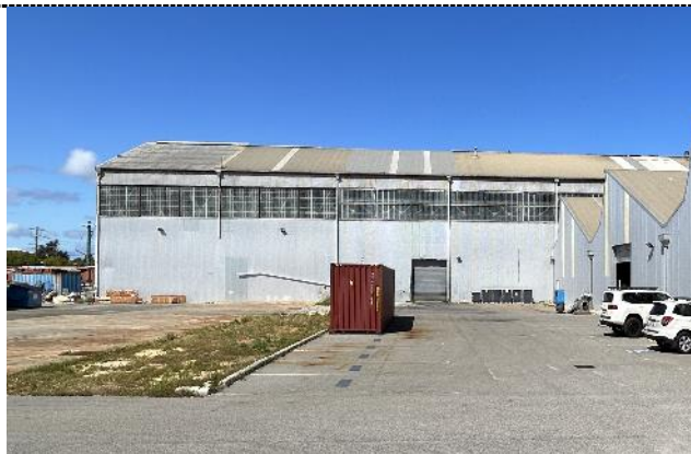
Figure 18. The full length double height warehouse building along the southern edge of the site has a gable roof clad in a variety of corrugated sheeting. Walls are corrugated metal sheeting with high level windows. The form of the windows reflects those on the southern side in that the majority of the panes are the larger rectangular shape with the last two bays having smaller panes.
