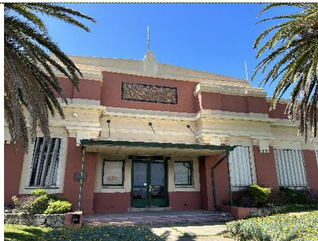
Figure 11. The main entrance is marked by a simple and stripped back cantilevered canopy, attached to the facade by structural tie rods. The entry element stands proud to the façade with decorative parapet, pilasters and horizontal pressed cement banding.
