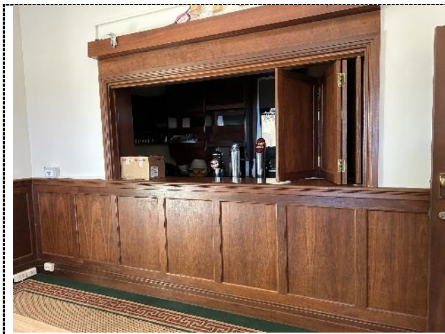
Figure 23. Non-original bar in the boardroom. The panelling reflects the original timber panelling of the building though does not match exactly with an increased width of panel in the later panels.
