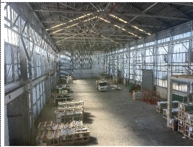
Figure 28. Southern warehouse, taken from the upper offices. The trusses are timber in the original section, while steel trusses have been used in the later addition. The timber trusses have been painted silver.
